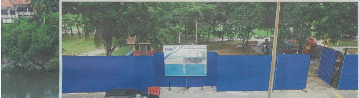
Hoarding surrounds the Pengkalan Batu Park that is under construction beside Sungai Klang.
