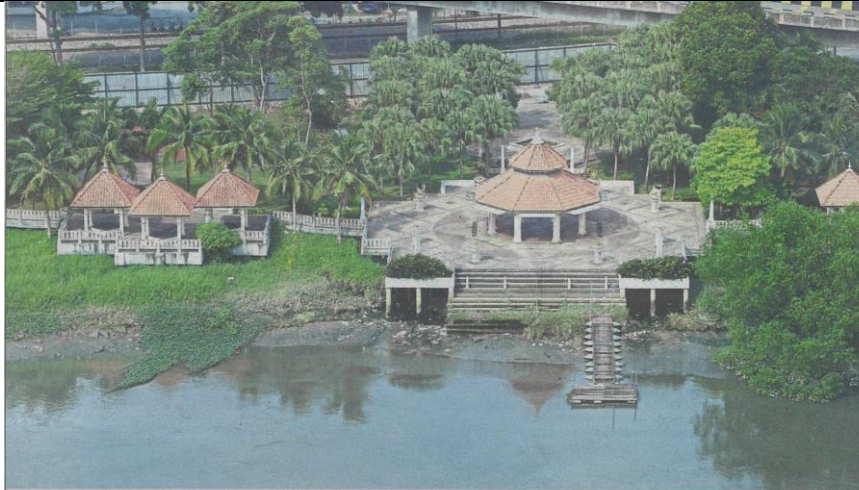
Ongoing redevelopment of the Pengkalan Batu Park, located along Sungai Klang. — Photos: KAMARUL ARIFFIN and IZZRAFIQ ALIAS/The Star
